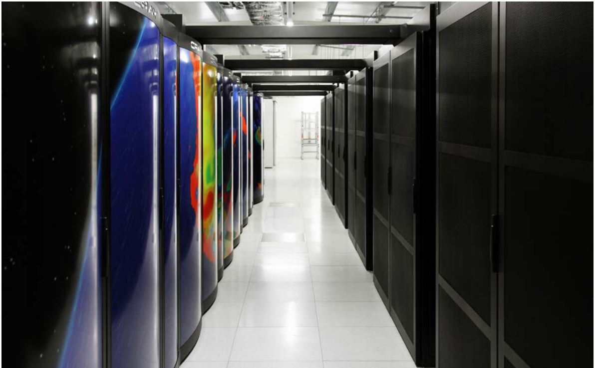
Figure 6. HPC 3 Data Hall Interior. Photograph by the author (2022).
