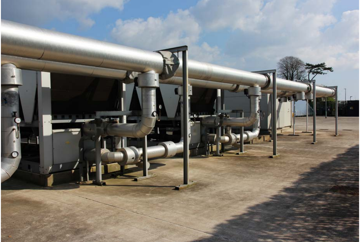
Figure 5. The air chiller units for the HPC Facility. Photograph by the author (2022).
