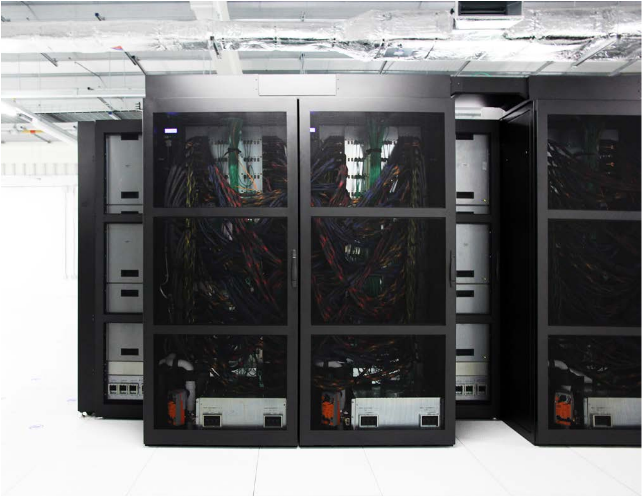
Figure 1. The Met Office HPC 3 Cray XC40 system, view of rear data and cooling. Photograph by the author (2022).
